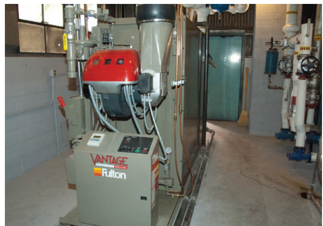
Vantage Hydronic boiler for the District 9 office.
