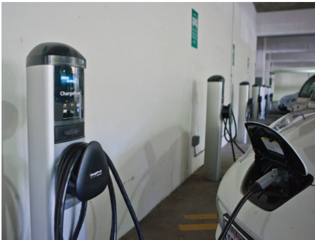
Electric vehicles charging at a parking lot facility.
