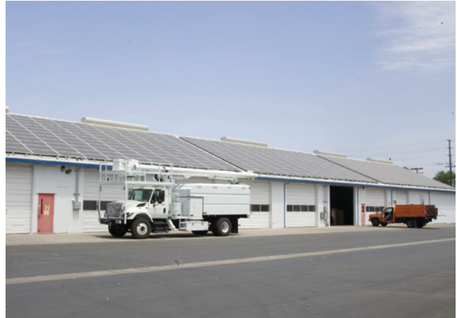
Solar panels on roof of District 10 equipment shop.
